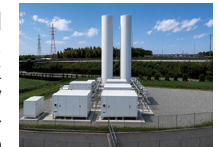
PEM water electrolysis demonstration unit at the Nishio Die-Casting Plant (rendering of completed unit)
