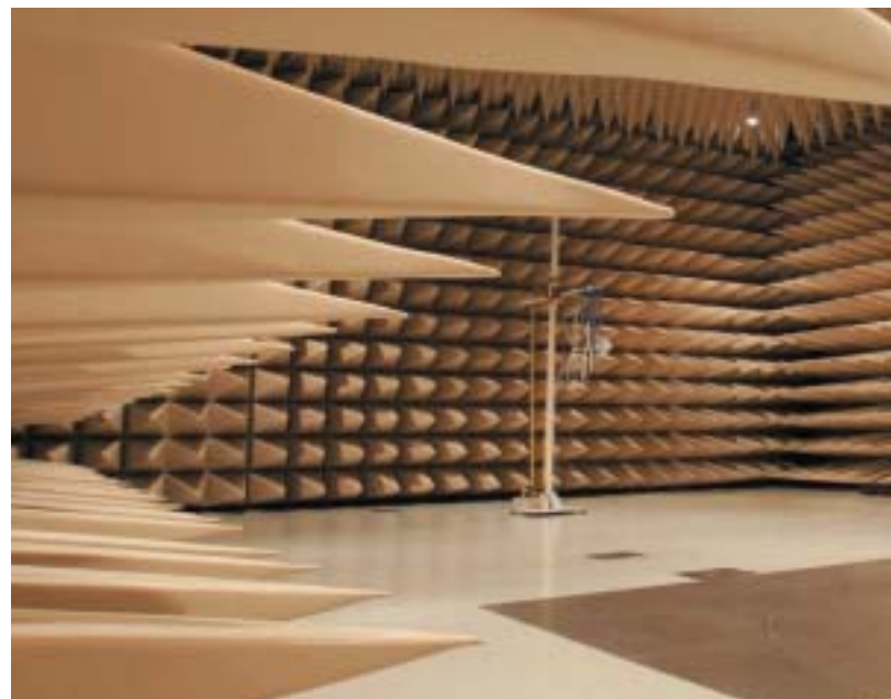
Anechoic chamber which evaluates the influence of electromagnetic waves, ranging from low to high frequency zones, on electronic devices
