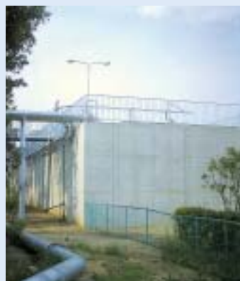
Waste Emission Emergency Storage Tanks (Nishio Plant)
